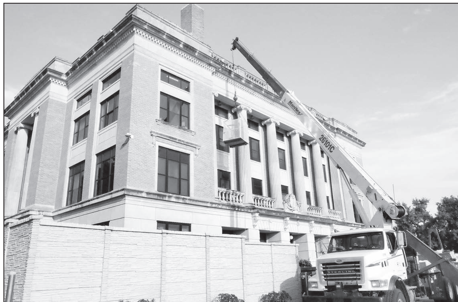
A new roof was installed on the Jackson County Courthouse after it was damaged by hail earlier this spring. A crew from Midwest Coating of Topeka hauled materials onto the roof with a crane located on the east side of the Courthouse. The Midwest Coating crew also attempted to check on an inoperable light bulb near the top of the building in this photo, taken on Tuesday, Sept. 22.
