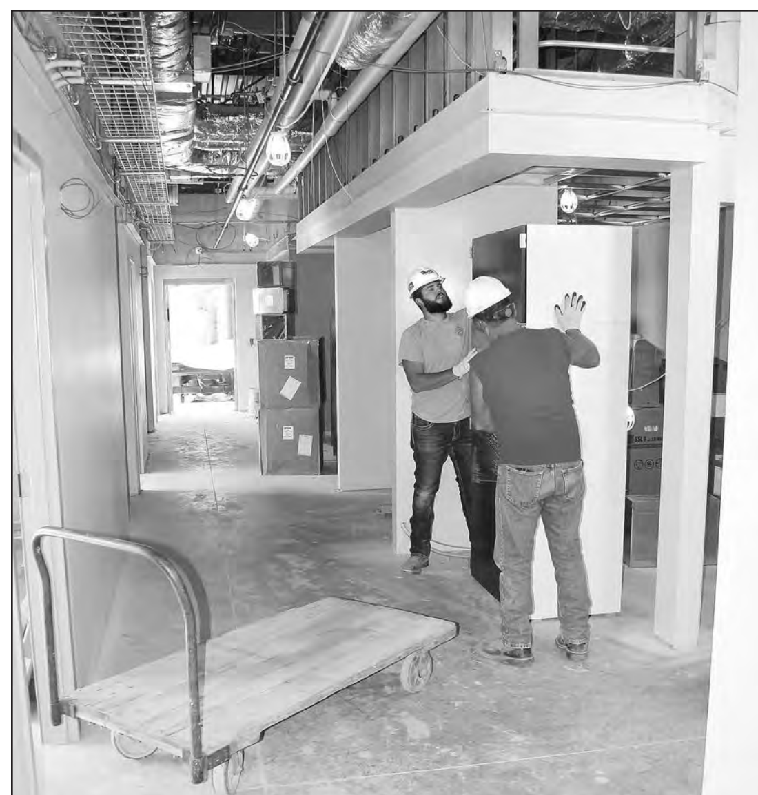
Logan Scheidel (left) and Dirk DeKoning of AHRS Construction recently prepared a cabinet for placement in one of the offices at Holton Community Hospital's new rural health clinic...
