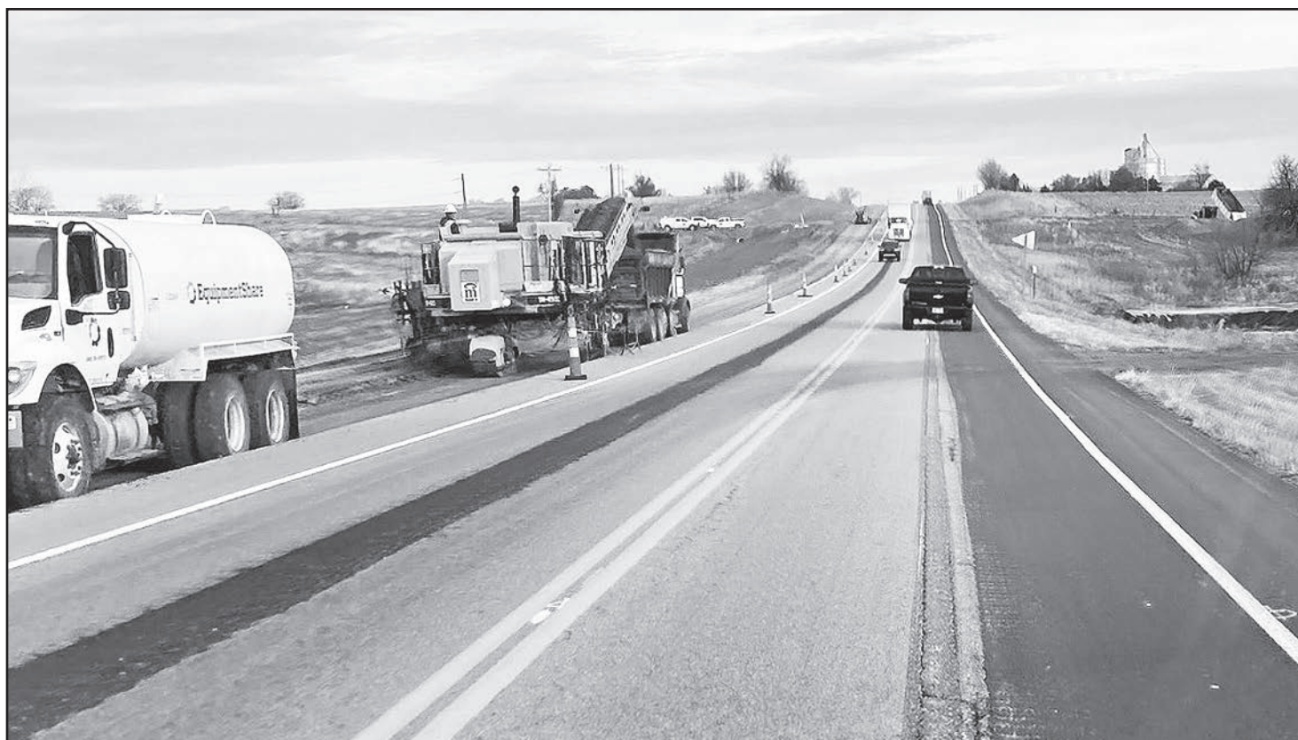
In the photo above, looking north toward Netawaka, construction work on the southbound passing lane along U.S. Highway 75 south of Netawaka is nearing completion, with all work on passing lanes in north Jackson and southern Brown counties expected to be completed by this coming spring, according to a Kansas Department of Transportation spokesperson.
