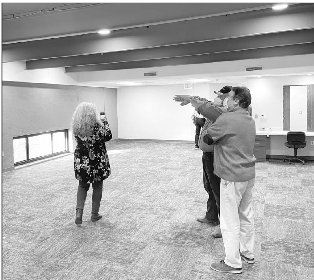
Construction of the new offices for the Jackson County Attorney and staff is almost finished on the fourth floor of the Jackson County Courthouse. In the photo above, Jackson County Commissioners Janet Zwonitzer (left) and Ed Kathrens (center) and newly elected Commissioner Dan Brenner (at right) viewed the new office space during Monday's commission meeting. Years ago, the space served as the Jackson County Jail, and most recently, it had been used for storage by several county departments.
