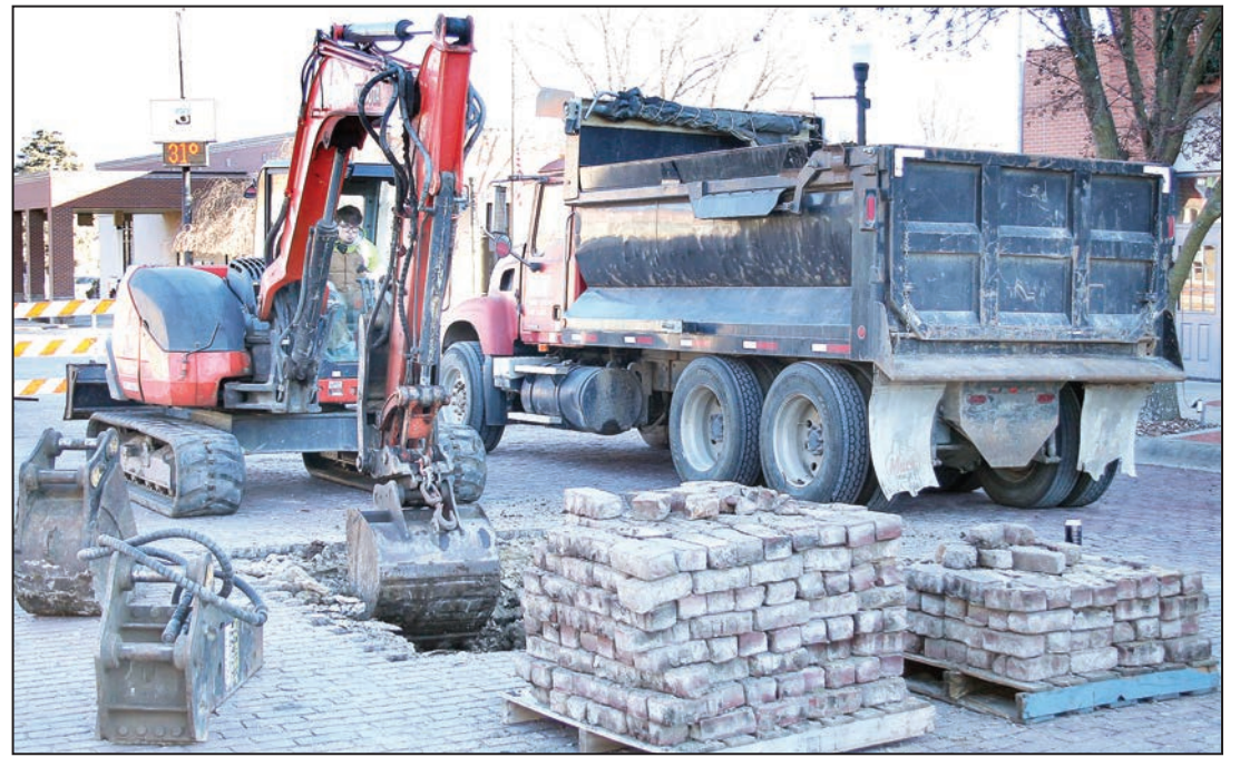
Chris Lewis of Hiawatha’s Jadwin Construction and Development dug his way into Pennsylvania Avenue on the east side of Holton’s Town Square on Monday morning in preparation for installation of a new manhole near Holton City Hall.
