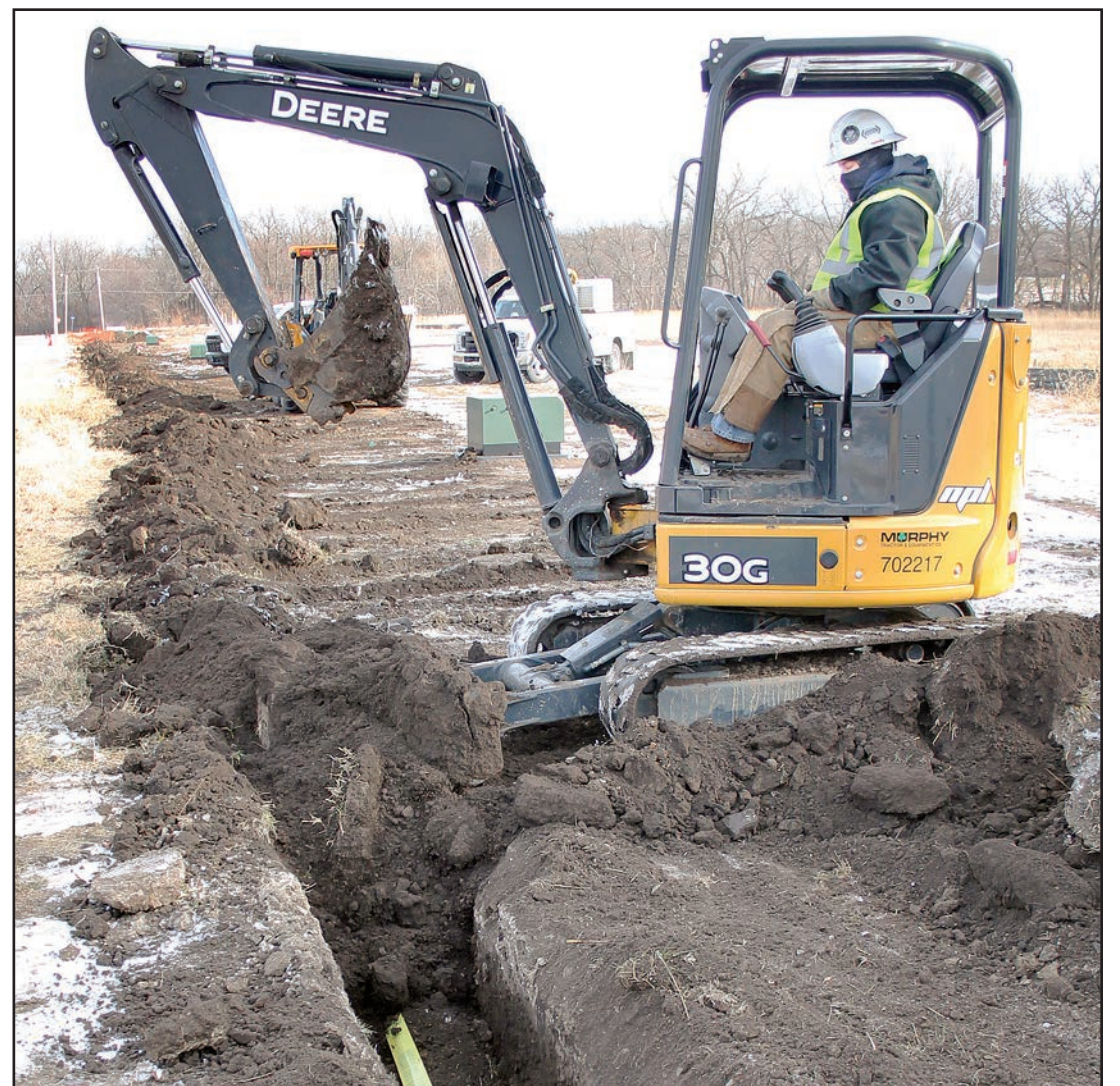
Preparation work continues at the new Banner Oaks subdivision on Banner Road in Holton, and on Friday, Patrick Gilliland of Topeka's Northern Pipeline company could be seen covering up a natural gas line that had been installed earlier for use in the subdivision.
