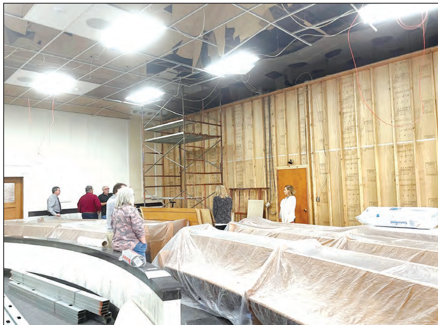
Renovations to the district courtroom on the third floor of the Jackson County Courthouse are under way. In the photo above, the Jackson County Commissioners and other county employees met with Mike Tindell of Coal Creek Construction of Auburn to discuss the project. A change order was recently approved to restore original architectural features of the room next to the ceiling, which have been covered up for many years. Photo by Ali Holcomb
