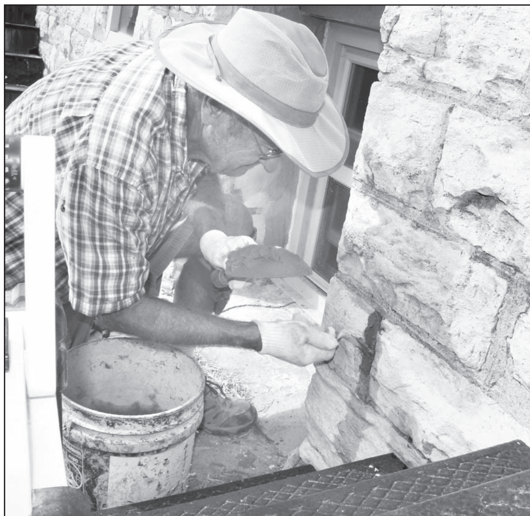
Gary Salts of Holton spent a recent morning on an ongoing project: using concrete to fill in cracks in the brick walls along the side of the Kellerman Insurance and Real Estate building. Photo by Brian Sanders
