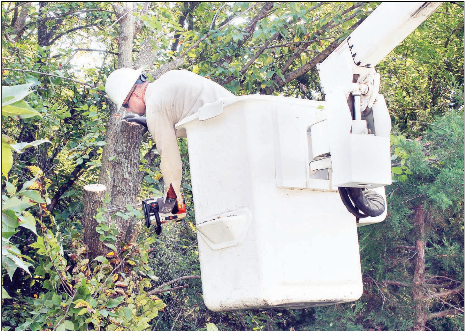
Holton city employee Andrew Hinman took to the bucket truck Thursday morning and used a chainsaw to cut limbs from trees along Q Road (Old U.S. Highway 75) south of Holton, just north of 214th Road. The trees were getting a trim as part of Holton's ongoing efforts to cut limbs and branches away from city power distribution lines, which stretch outside the Holton city limits. City Manager Kerwin McKee said the city's power lines extend about three miles outside the city in all directions, and trimming trees and brush near the lines is one step the city takes to lessen the possibility of broken power lines due to fallen limbs and branches.
