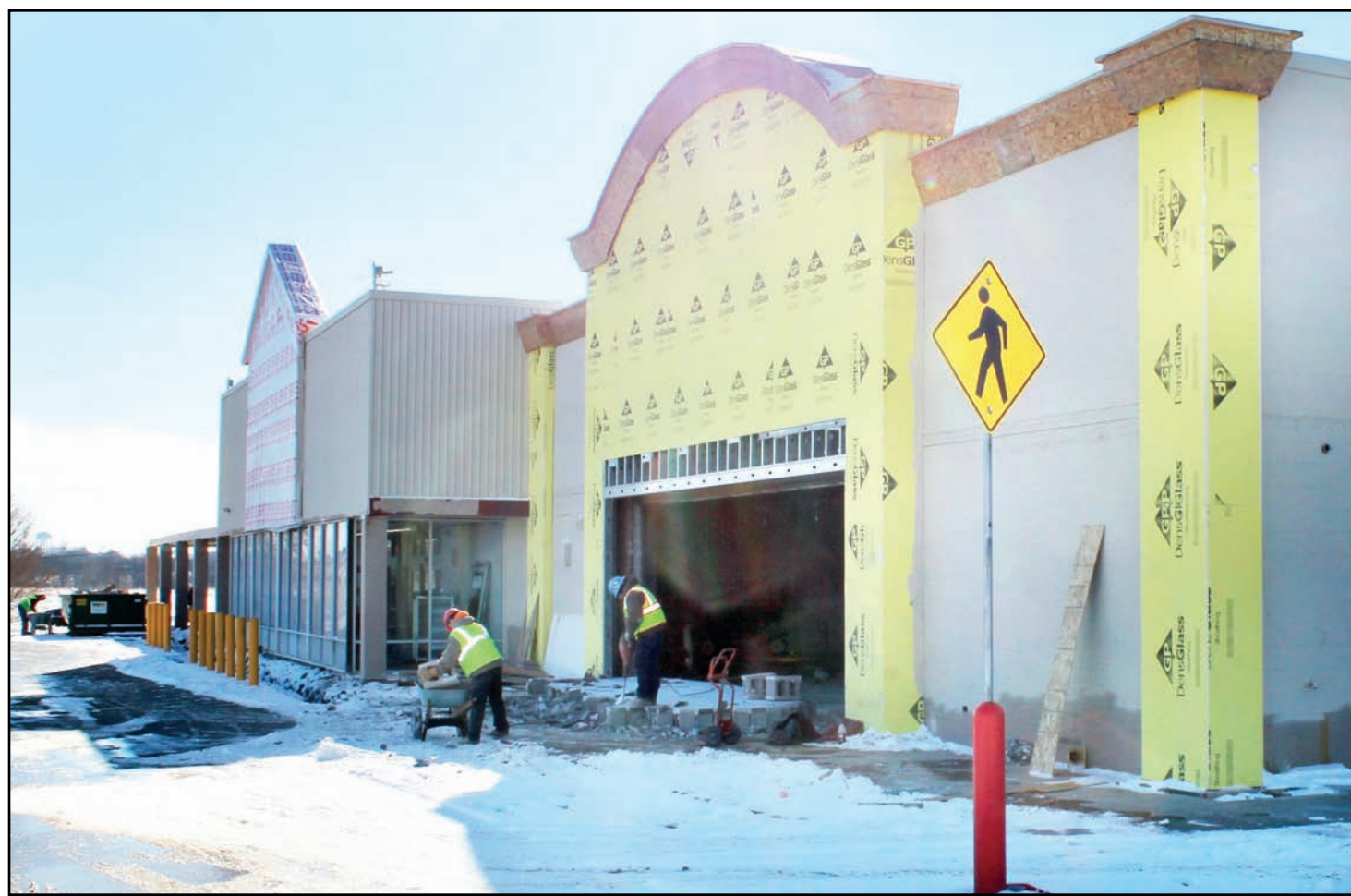
In spite of cold temperatures, crews continued to work Friday on splitting the old Holton Walmart building for the upcoming opening of new Tractor Supply Company and Dollar Tree outlets here. Building permits were issued in December for each of the new stores, which are expected to open later this winter.
