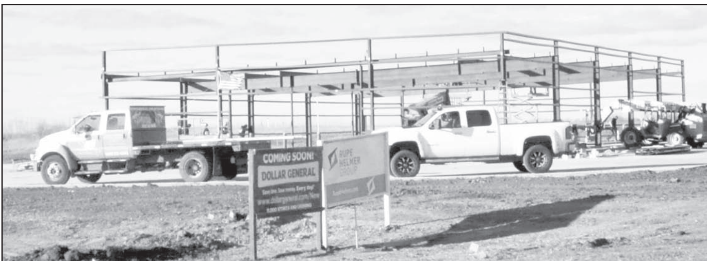
A new Dollar General is being built in Hoyt at the intersection of U.S. Highway 75 at 110th Road. New "built-to-suit" Dollar General stores range between 9,000 to 9,500 square-feet on approximately one to one and a quarter acres of land, it was reported. The new store is being built by the Rupe Helmer Group. Photo by Ali Holcomb
