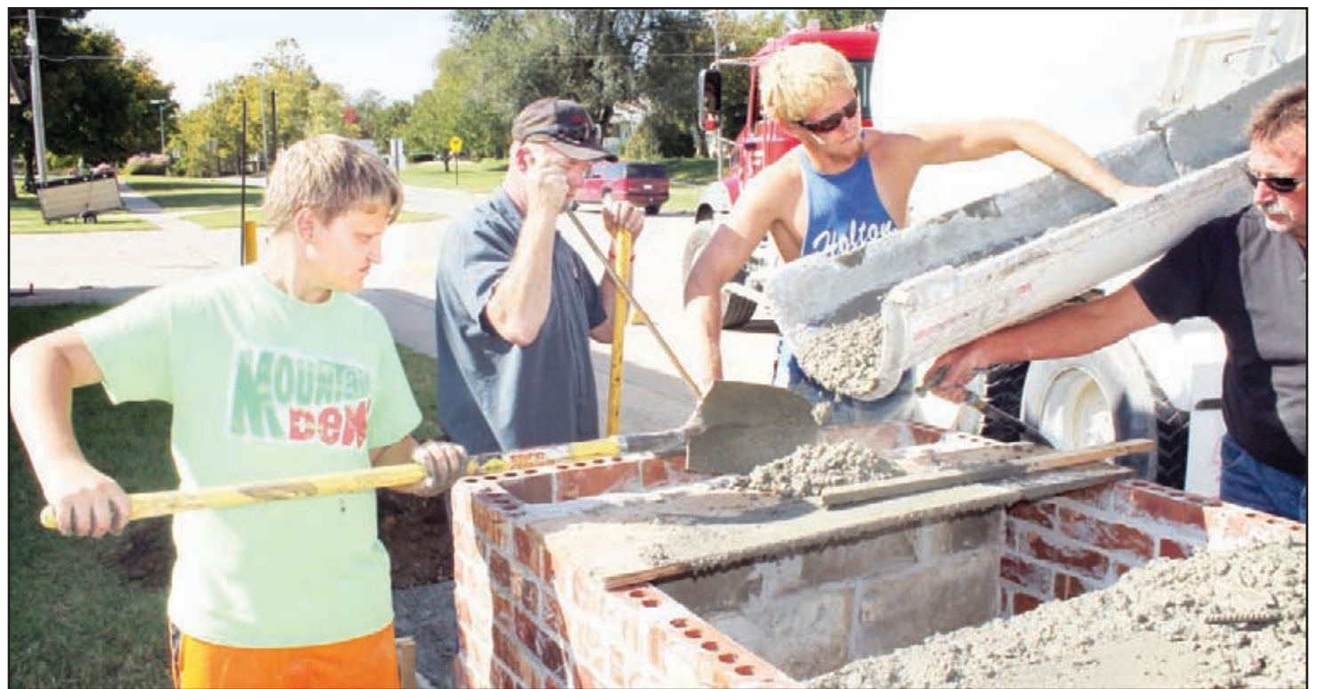
Kyle Figge (left) got some assistance from Mark Sullivan (right) and Lane Slocum (second from right) of Sullivan Construction of Holton, as well as John Motto (second from left) of the Holton Fire Department, in pouring concrete Tuesday afternoon at the Holton Public Safety Building for the base on which the old Linscott bell will be mounted in the near future, as well as concrete for the bases of two flagpoles that will be installed near the bell mount. The work is part of Figge's Eagle Scout project, which involves the mounting of the old bell that dates back to the old S.K. Linscott Farm in 1889 on the base at the Public Safety Building. Figge's father, Holton Boy Scout Troop 64 scoutmaster Craig Figge, said Veterans Day has been set as a tentative unveiling date for the bell mount. Photo by Brian Sanders
