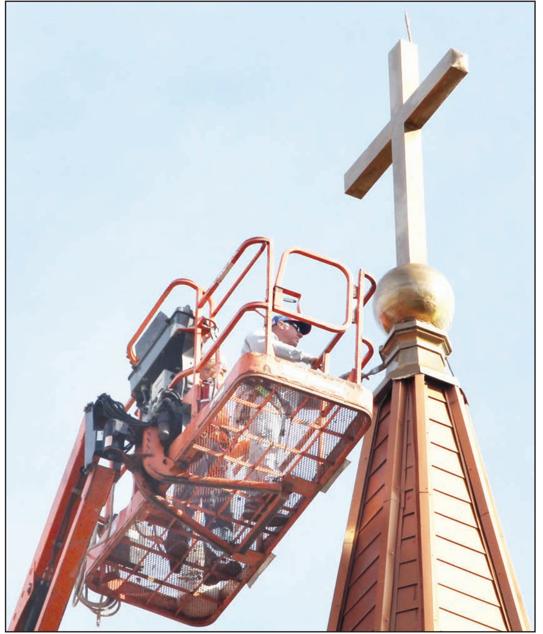
Robert Tharp (right) and Rufus Schaver (left) of Heinen Custom Operations added a coat of paint to the cross and portions of the steeple at St. Dominic Catholic Church in Holton on Tuesday. Last week, the company replaced the vented louvers on the sides of the church.
