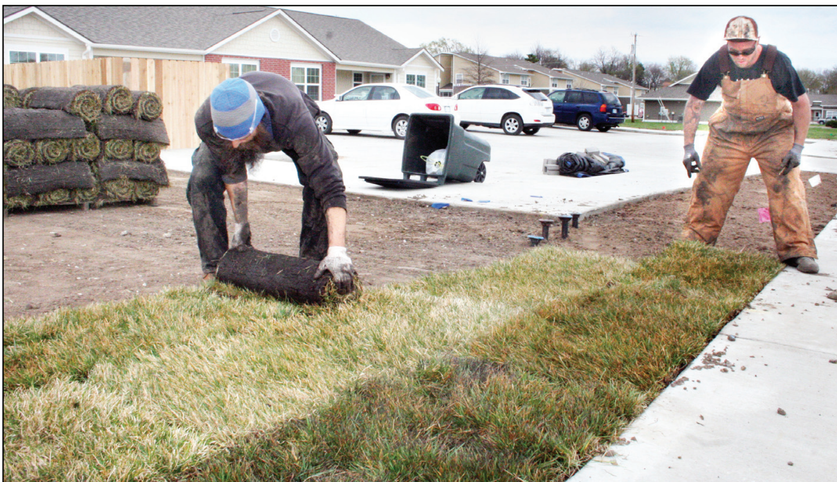
Eric Tweeten (left) and Derek Beerbower, working for Tree-Riffic Landscaping of Wichita, were among those busy laying out rolls of sod at the Prairie View Senior Residences housing complex on Tuesday afternoon. The landscaping crew said it is likely that laying sod and seeding will continue into next week. Tom Bishop of Homestead Affordable Housing said the new, 32-unit senior housing complex recently received its final certificate of occupancy.
