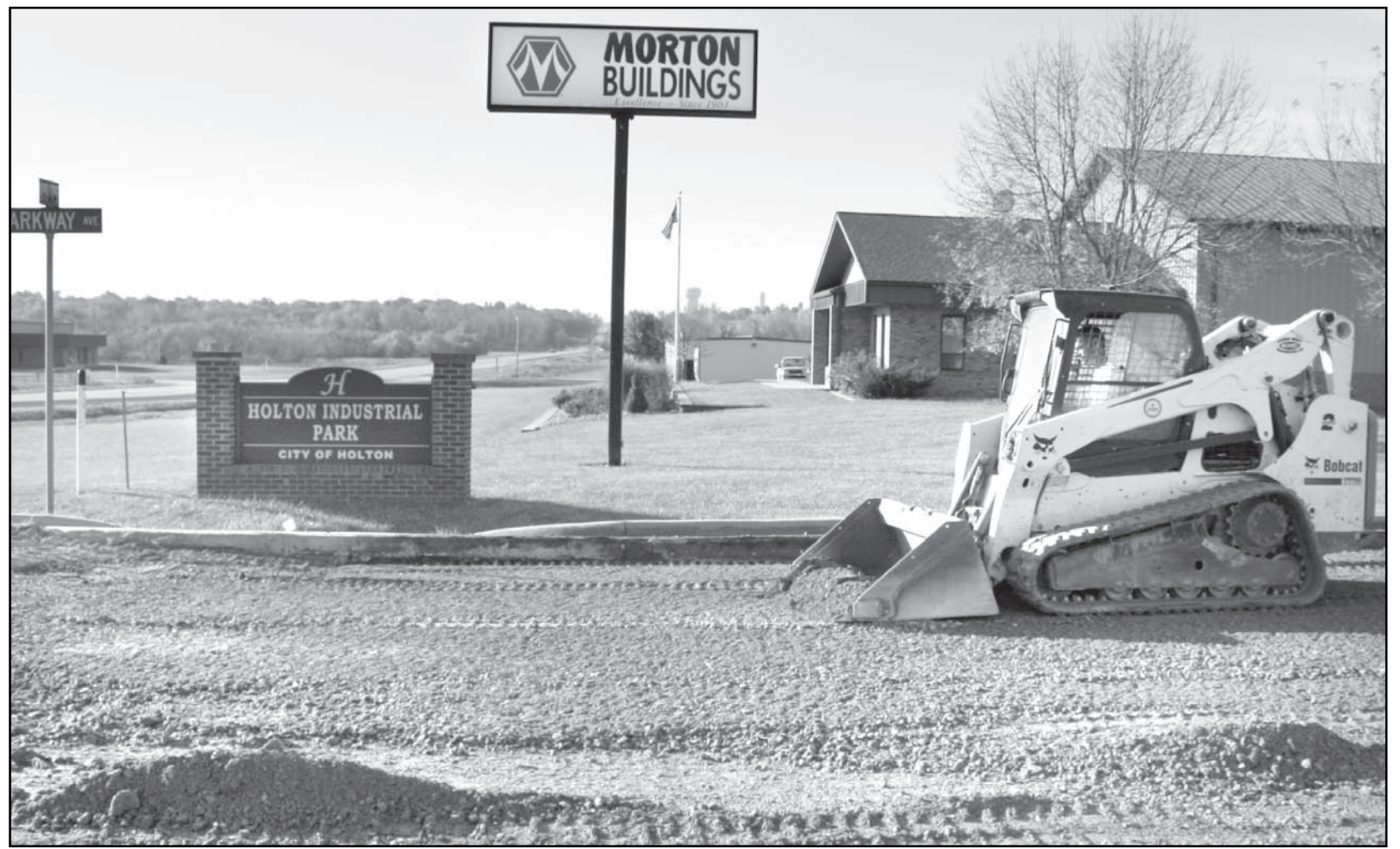
Doug Dixon of Kansas Heavy Construction Inc. of Topeka spread base rock along Parkway Drive at the Holton Industrial Park in preparation for pouring of concrete sometime in the next few days. Bruce Rinkes of Holton's King Engineering, which is overseeing the Industrial Park road reconstruction project, told the Holton City Commission on Monday that all work on the road reconstruction project should be finished shortly before Thanksgiving.
